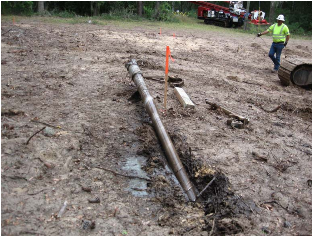
The bore tunnel for the HHD was thirty feet below Archers Creek and spanned its entire length. The above picture shows the accuracy of where the drill came out in relation to the orange marker target.
